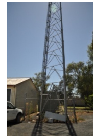
Figure 5 Existing communications tower to be retained
